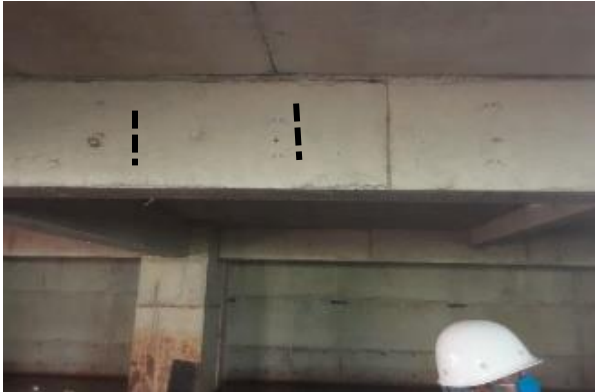
Figure 8: Crack patterns of the beam.
