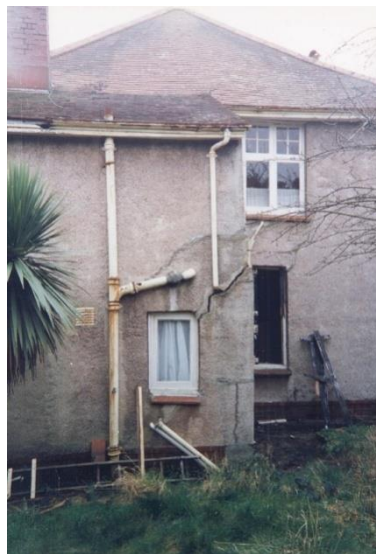
Figure 1: Cracked wall due to collapsible soil (Culshaw and Jefferson, 2018).
